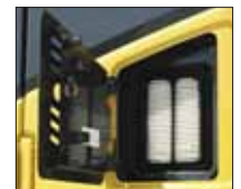
External air conditioner filter
